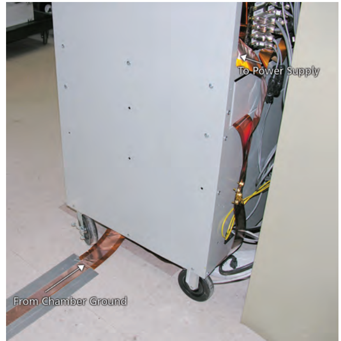
Figure 7. Copper ground strap leading to the power supply from the vacuum chamber
