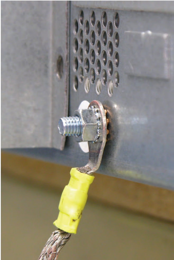
Figure 2. Crimped and soldered ground connection, made to unpainted surface
