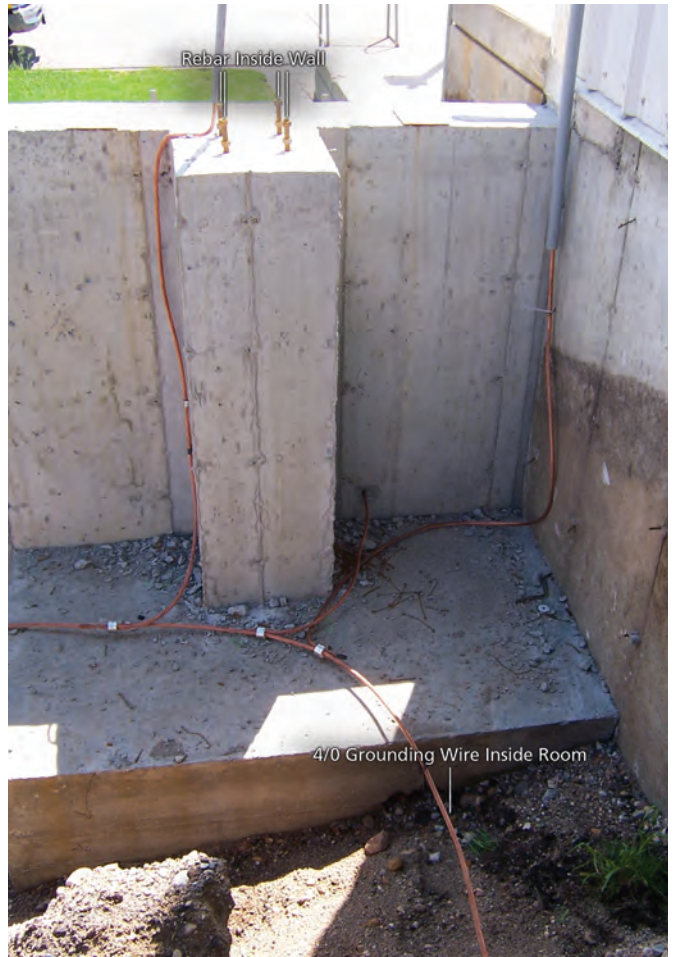
Figure 13. Room grounding wire connections to rebar inside wall
