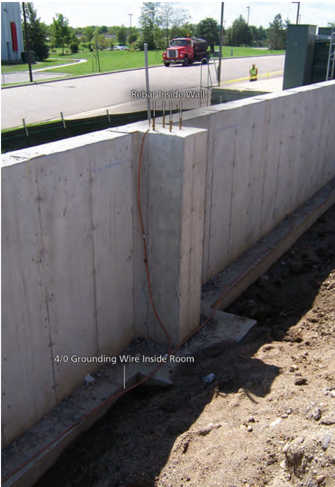
Figure 12. Room grounding wire connections to rebar inside wall
